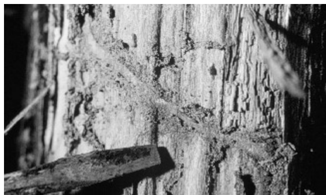
Figure 3-8. Termite-damaged wood. A mud tube has been opened, exposing a worker termite.
