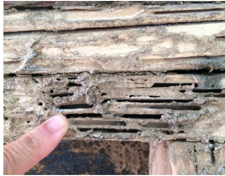
Termite damage under a window frame. Notice the galleries with the grain are packed with mud.
