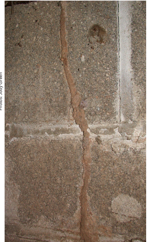
Mud tube running from soil in crawlspace over foundation block to the wooden sill plate.
