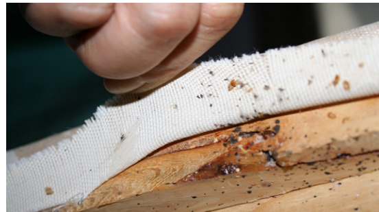
Bed bug spots under fabric stapled to the framing of box springs.
