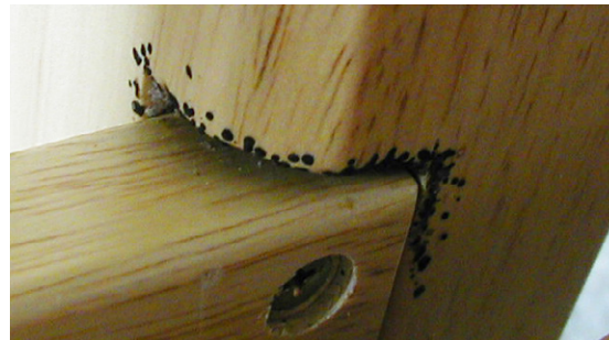
Bed bug spots near cracks of futon frame.
