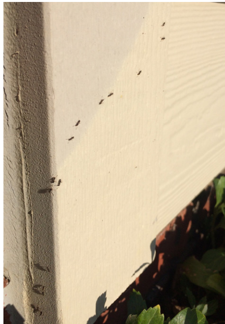
If you have ants indoors, look around your exterior foundation for trailing ants.
