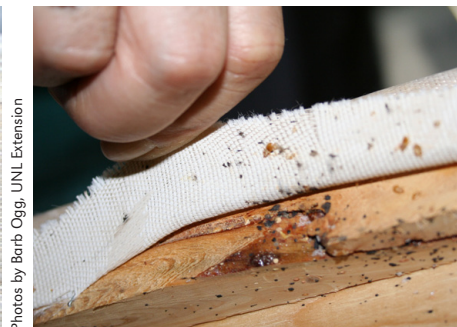
Bed bug spots under the fabric stapled to the framing of foundation/box springs.
