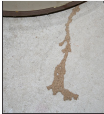
In February 2009, homeowners noticed termite mud tubes emerging from a crack in the basement floor.
