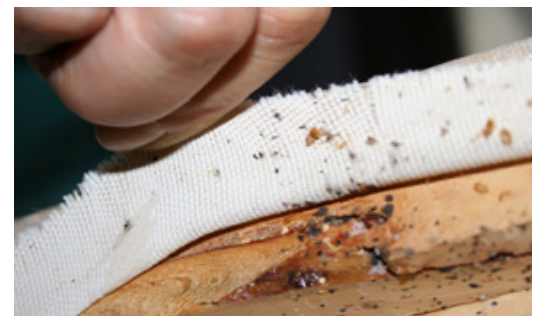
Bed bug spots under fabric stapled to the framing of box springs.
