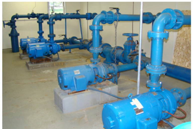
Pumps at one of five booster stations
