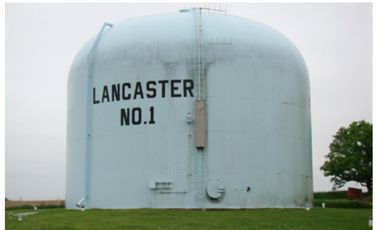
500,000 gallon ground-level storage tank
