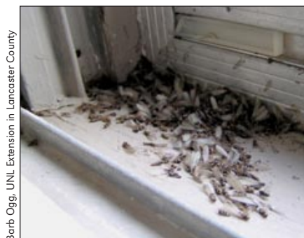
Dead termite swarmers in a window sill.
