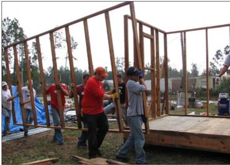
Each year UNL students share skill during their school breaks. During the January break, several UNL students helped build homes for hurricane victims in Hancock County, Mississippi.
