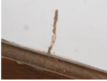
Mud tube on a basement wall
