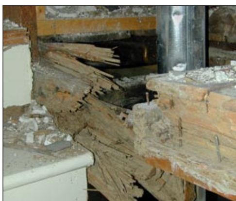
Figure 2. Termite damage to floor beam.
