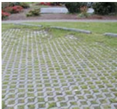
Porous (permeable) pavement allows rain to permeate the soil and gravel layers below.
