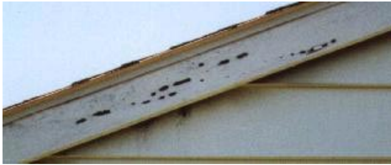
Woodpecker damage due to foraging for carpenter bee larva on fascia boards of a house.
