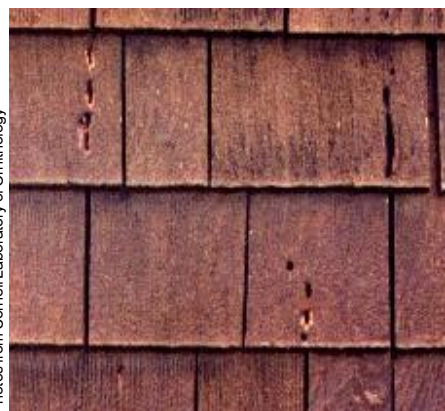
Damage due to woodpecker foraging for insects on cedar shingles.
