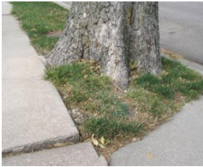
A tree located in south Lincoln — lateral growth of the tree roots is causing uneven displacement of sidewalk sections.
