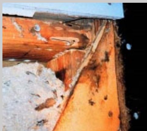
Carpenter ant nest in cellulose insulation inside exterior wall below window
