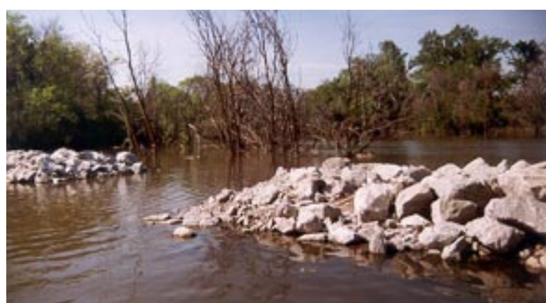
This in-lake sediment and nutrient trap was installed above Wildwood Lake in December 1993 and provided a model for similar structures in Olive Creek Lake and Wagon Train Lake.
